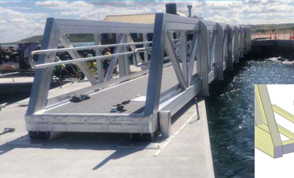
Tas Ports – 30m gangway with bump stops
